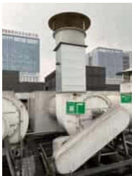
1#排气筒及活性炭箱
